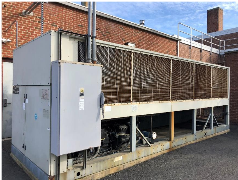
Figure 5: MSHS - 170-ton Air-cooled Chiller
