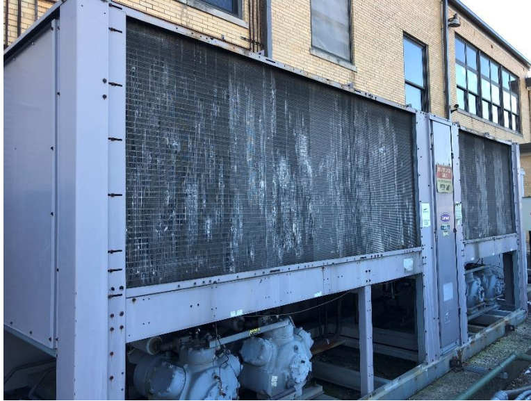
Figure 4: ES - 150-ton Air-cooled Chiller
