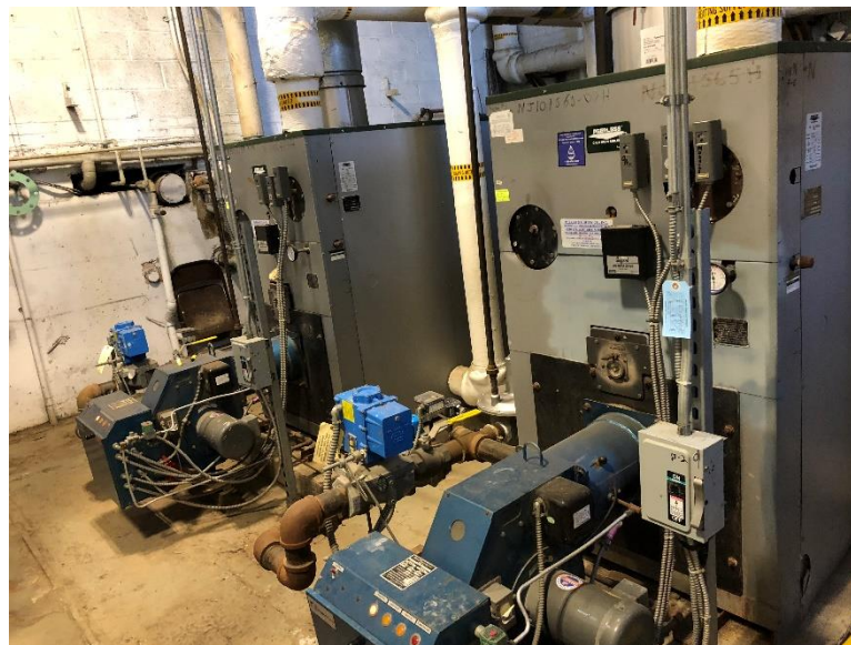
Figure 2: ES - Two (2) 4,663 MBH Gas-Fired Boilers
